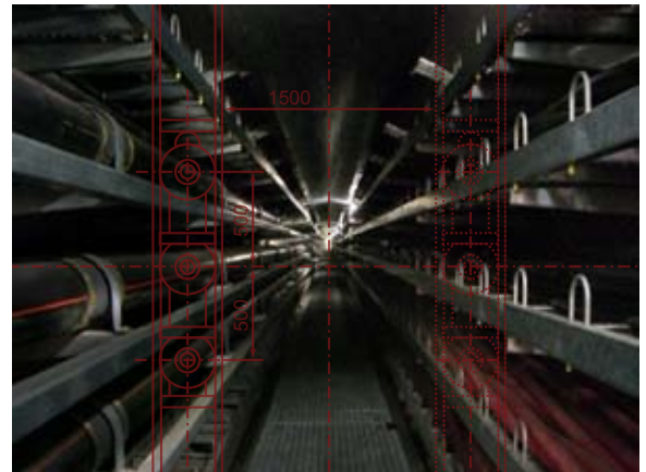
Installed cable system
